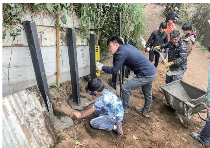
Micro-practice with local people to mitigate erosion by building piling walls in Barrio Cantera, an informal settlement with landslide risk in San Martín de los Andes, Argentina. October 2018.
