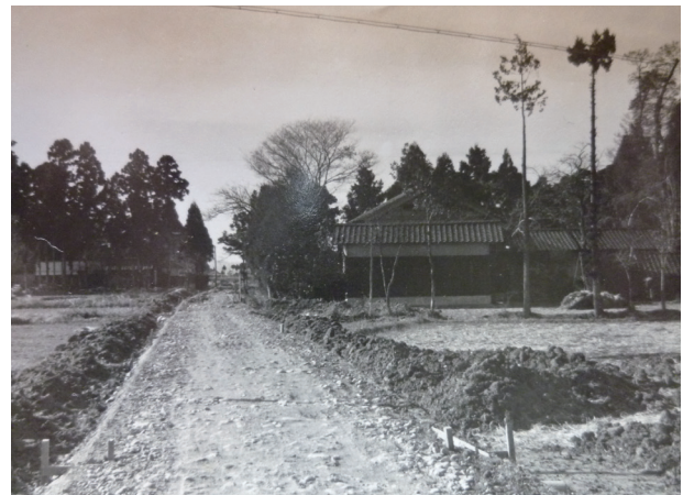
Photo 2. Village road construction in progress (Showa 30 period) Photo is provided by NAKAJIMA Katsutoshi
