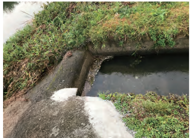
Photo 6. Umankashira nogoshi . The overflow portion has concrete block pitching to resist damage.
