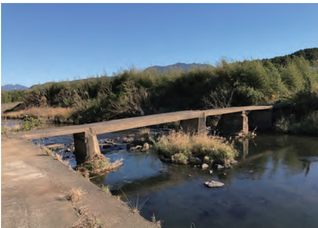
Photo 2. The Okawano flood submerging bridge
