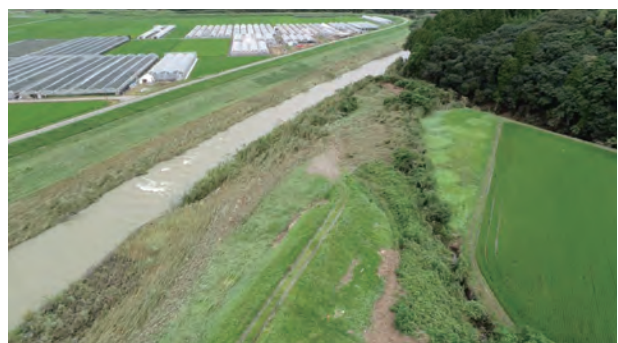
Photo 5. Floodplain open levee opening after a flood
