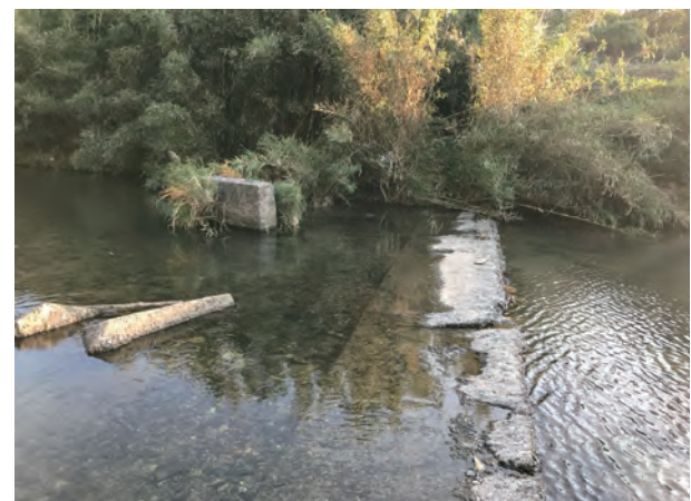
Photo 11. A flood submerging bridge with collapsed girders
