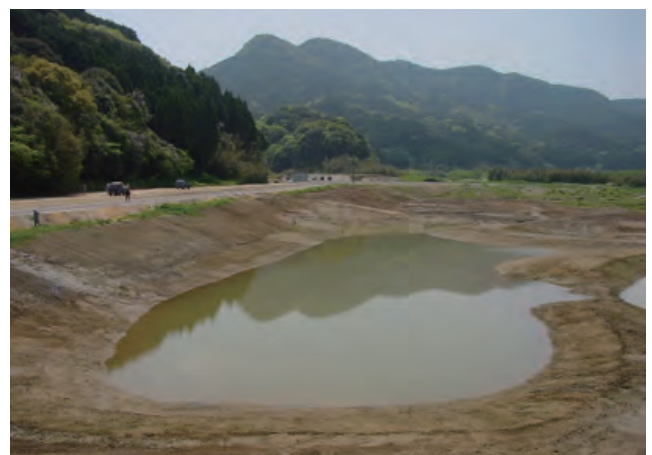
March 2004 Immediately after work: The body of water in the foreground is Shitaike. When excavation started, the land was barren without any vegetation.
