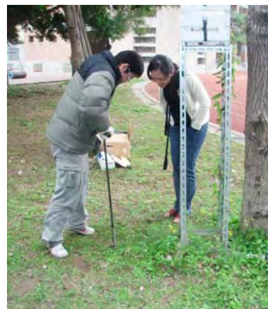
Fig. 4. Drilling of a slim hole for installation of soil temperature sensors beside a thermal recorder for air temperature monitoring (Bai, 2009).
