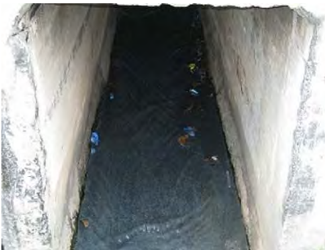
Pic.6 Sewage water pipe
