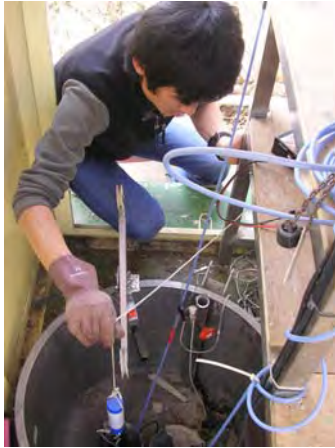
Fig. 8. Installation of water temperature recorders in an observation well in Taiwan.
