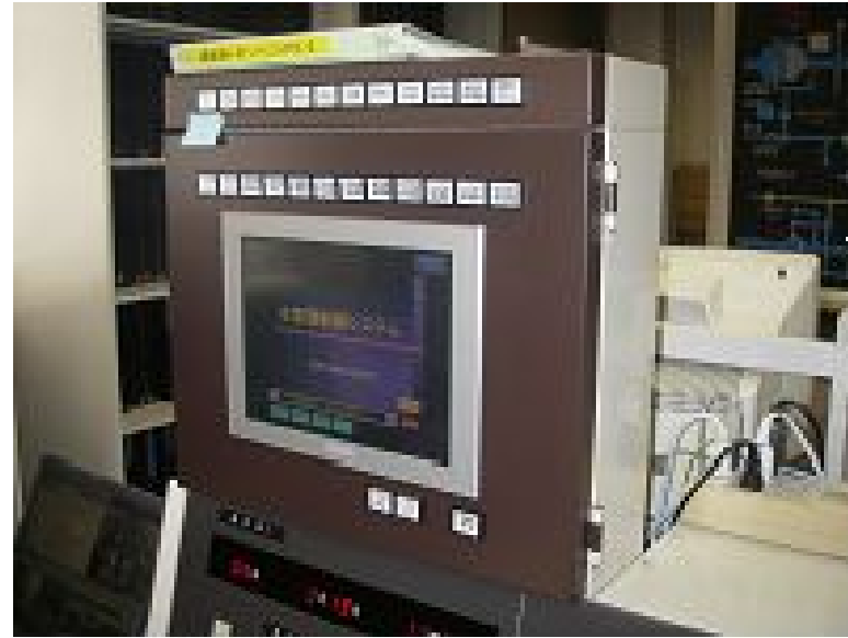
Operation panel of telemetry system
