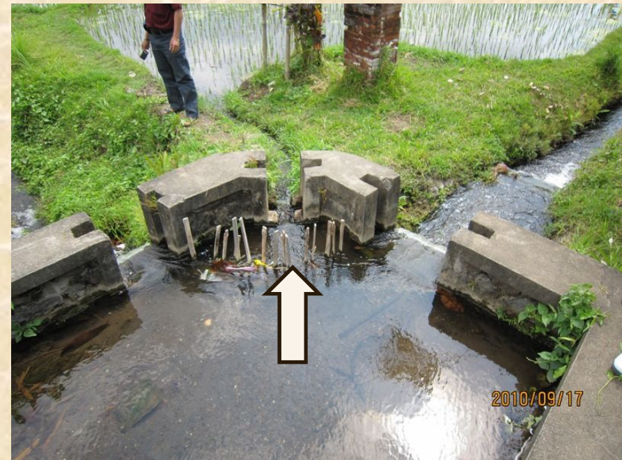
Division structure and a tertiary off-take: tek-tek is the base unit of water division in subak.
